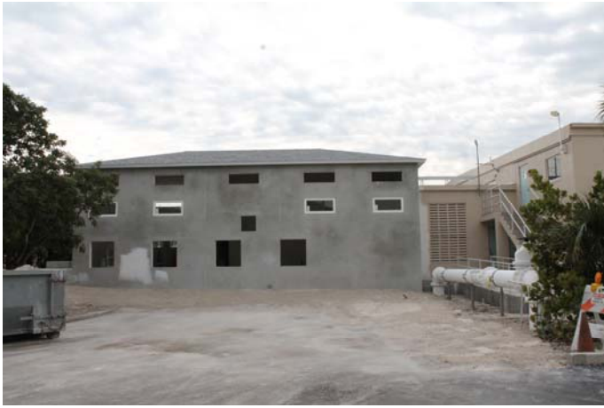
Northern View of Distribution Pump Station Addition
