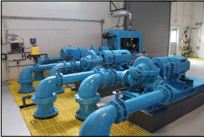
High Service Pumps in the RO Plant
