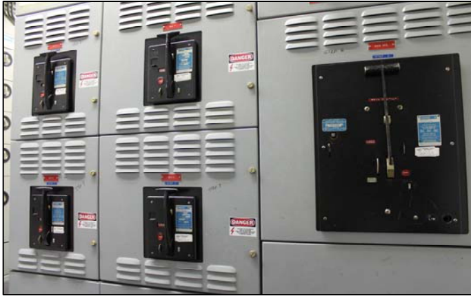
Four sub-breakers and one Main Breaker
