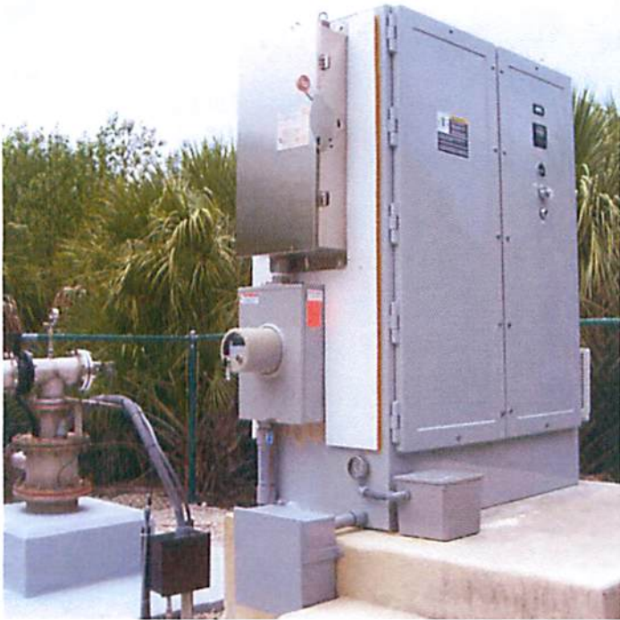
Suwannee Well 8 Control Cabinet
