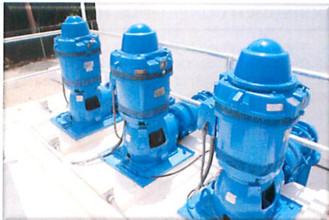
Existing Clearwell Transfer Pumps
