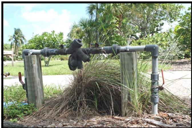
Typical Backflow Installation
